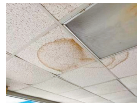
Royal Junior High School needs some ceiling repair work.
